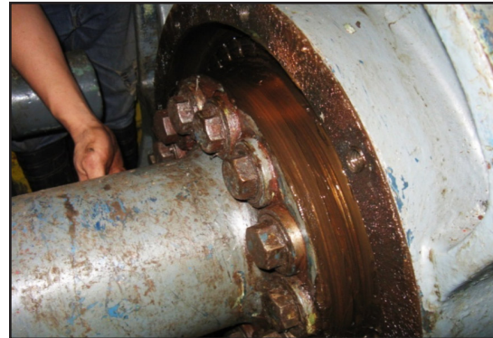
Previous grease did not prevent corrosion in wet conditions (red-brown rusty grease).
