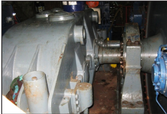
Thompson hoist for the man-lift is a safety component. Reliability is CRITICAL.
